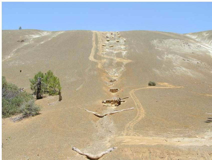
Photo 4. Polygon 25 barrens restoration. Note workers installing straw bale check dams near the top center of the barren for scale.
