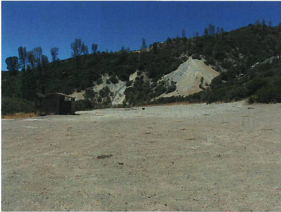
Figure 4. SA 1. Sediment averaging 8 inches depth covers half of the SA. Soils are compacted. Most of the sediment originated from T105 which departs from the SA up the slope to the right.
